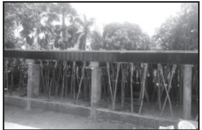
On going project of Prathna hall & Guest House construc- tion at Gandhinagar Temple
